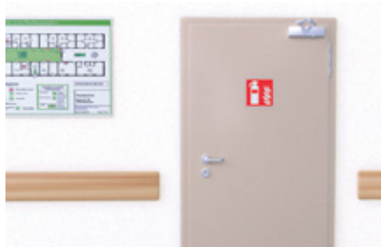
Fire protection doors
