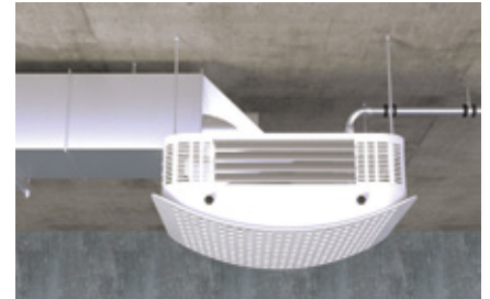
Air conditioning units
