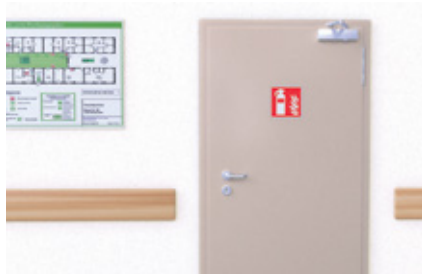
Fire protection doors
